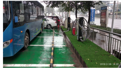
An electric bus being charged using a fast charging station at the Group's 4S service centre in Naxi County in Luzhou City
